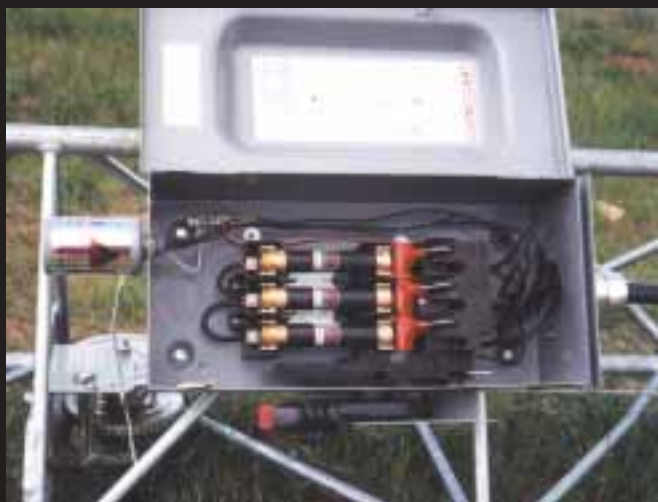
Overcurrent protection at the tower's base.
